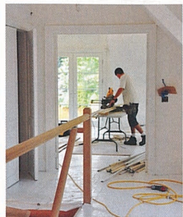
The house is abuzz with saws and drills as the construction crew and tradesmen move indoors to build the banisters, finish the trim and fit our custom pieces.
