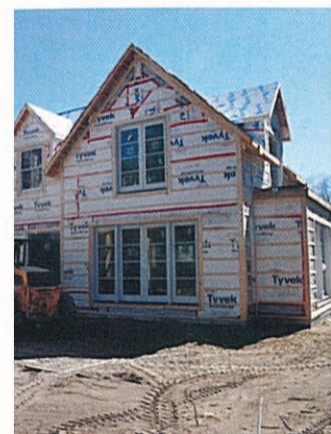
Months of planning on paper, the plans of the house finally go up, and we get to work fine-tuning the interior, favourite part of the process!
