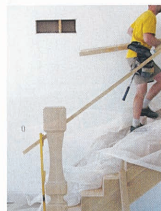
Stairworks/Flourish Design Elements custom-made the newel post. It gets a lot of oohs and aahs when it goes in and is the architectural moment we hoped for.
